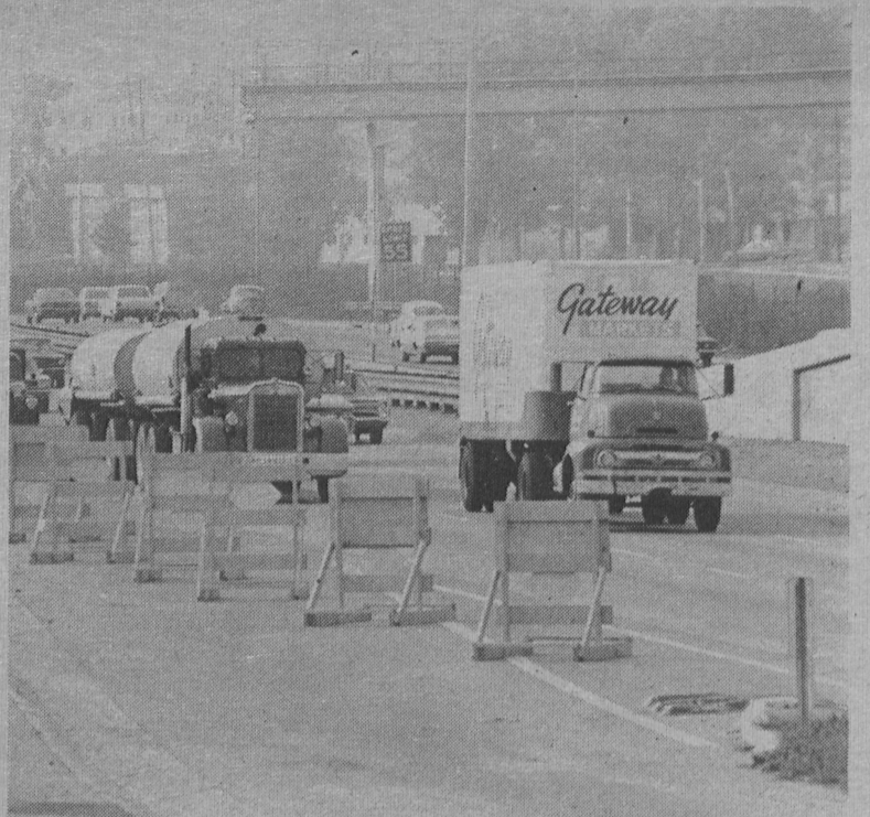
FREWAY CONSTRUCTION--- Work has started on the San Bernardino Freeway. Eventually, one lane in each direction will be added to facilitate traffic flow, planners say. Half-removed bridges present a picture out of the blitz. (C.T. Photo by Bob Weeks)
